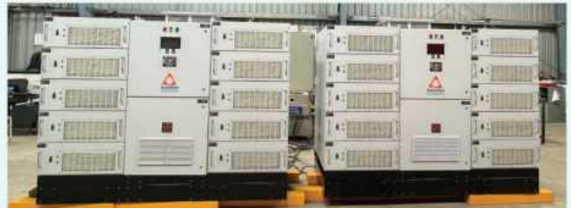
Composed of Two 1.25 MVar Systems each with 10 Modules in parallel
